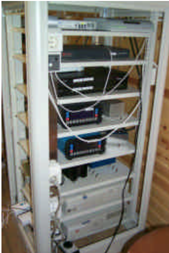
Figure 3.3: Interior of a complete SWEPOS station.
